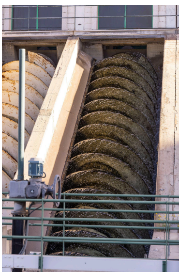
Figure 18: What is seen is an Archimedes screw, designed, when rotating, to lift water, fluids or solid materials (such as grain) from a lower area to a higher one. It consists of a
