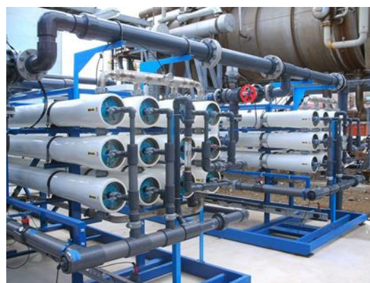
Fig. 3 : Pressure vessels and piping systems within a desalination plant on Curaçao.
