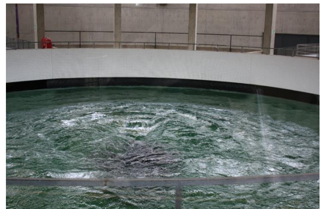
Figure 2: Swelling pot at the treatment plant of the Lake Constance Water Supply (BWV)
